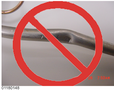
Figure 6-15 Damaged Capillary Tube
